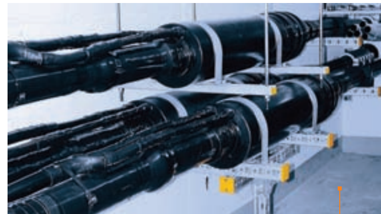
Laying in a tunnel: Joints with Cu-tube and HDPE-coating in a tunnel.
