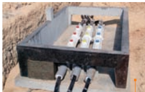
Laying in a pit: Joints with protection box in a concrete pit.
