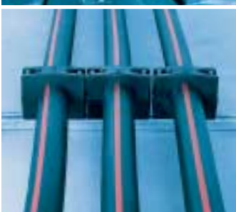
Good routing. Synthetic rubber clamps for fastening and alignment of cables to required route.
