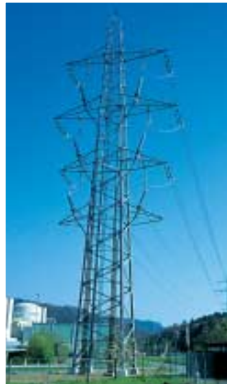
FR 1.245-01 Outdoor sealing ends with composite insulators mounted on pylons.
