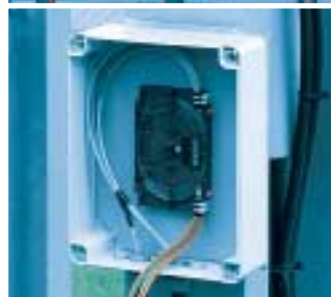
Temperature measurement. Sealing end box for temperature measurement by means of optical fibres in the cable sheath.
