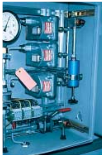
All under control. Pressure control box for oil-filled cables with pressure gauge, pressure switches and pressure pump.
