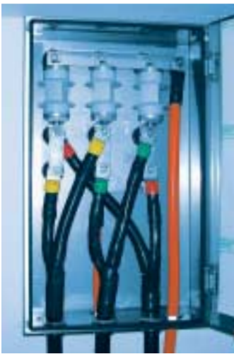
Cross-bonding link box. For the cross-bonding of cable screens. The surge voltage arrestors protect the outer sheath of the cable from both switching and atmospheric over-voltages.
